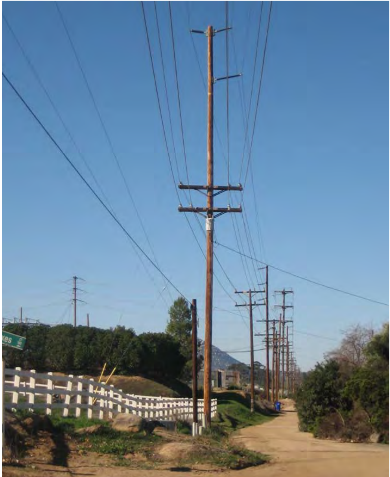
Typical wood transmission pole (with distribution underbuild)
